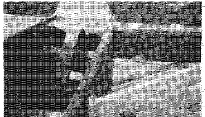
Lumber bondo'd from fuselage to centersection spar to firmly locate it while it is taped in place.
